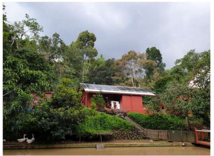
@ Bandung - 5 kW On Grid
