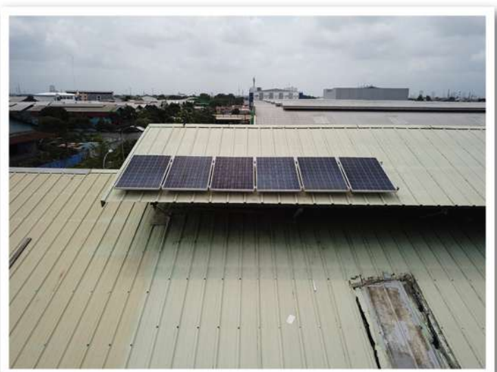
@ Daanmogot - 1 kW On Grid
