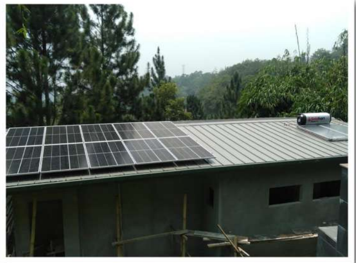
@ Bandung - 5 kW On Grid
