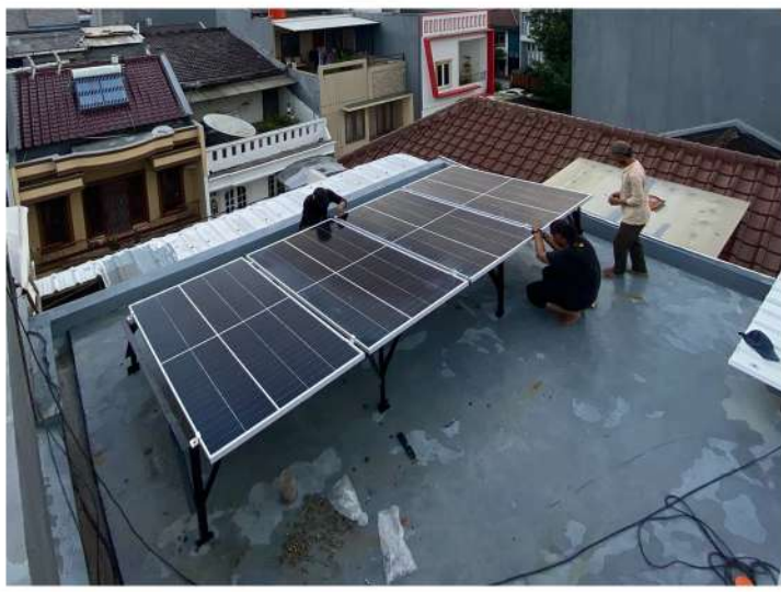
@ Sunter - 2 kW On Grid
