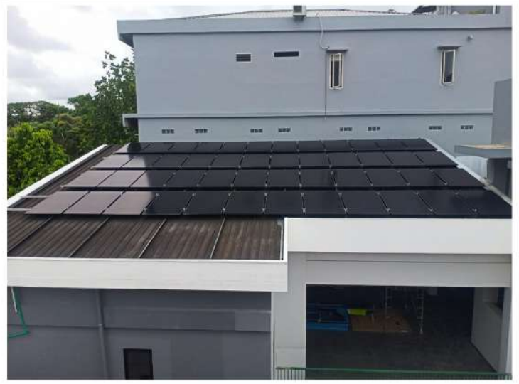
@ Ambon - 15 kW On Grid
