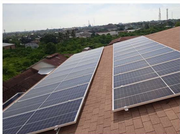
@ Ambon - 10 kW On Grid
