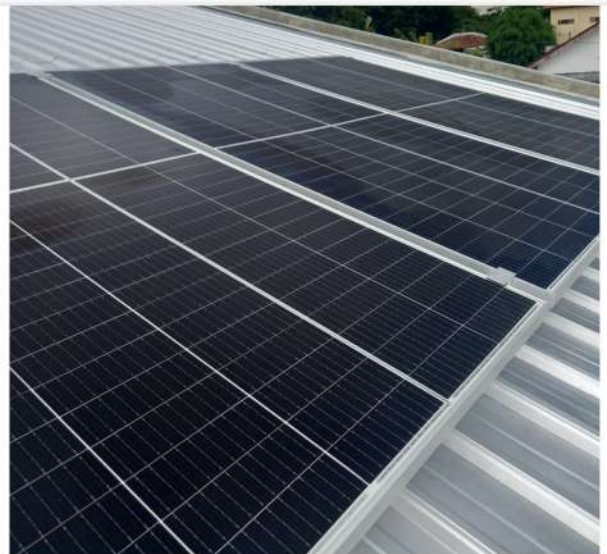
@ Klaten - 5 kW On Grid
